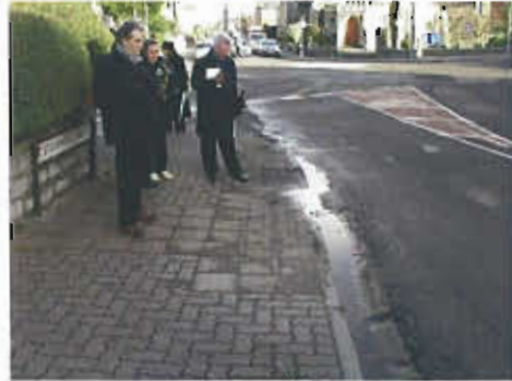
Stanwell Road poor detail at drop crossing
