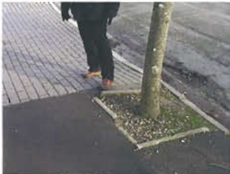
Grove Terrace Trip hazard at tree pit
