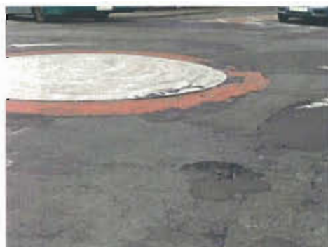
Stanwell Road etc roundabouts defects
