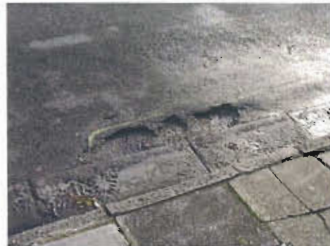
Victoria Avenue Pothole marked for attention some time ago
