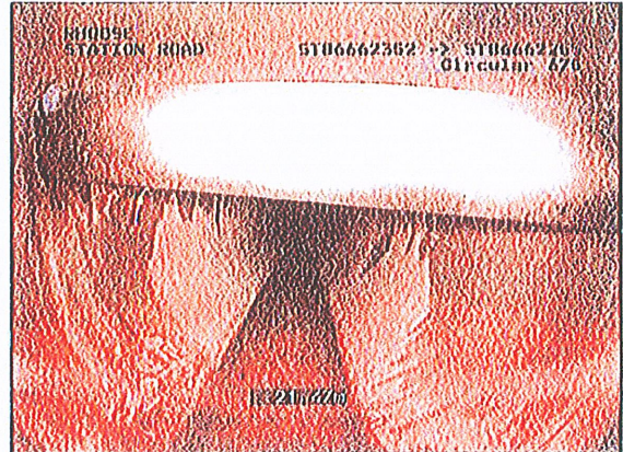
Photo: 14a, Tape No.: 01, 00:00:00 21.47m, Obstruction, 30 % height/diameter loss, Remark: PIPE THROUGH CULVERT
