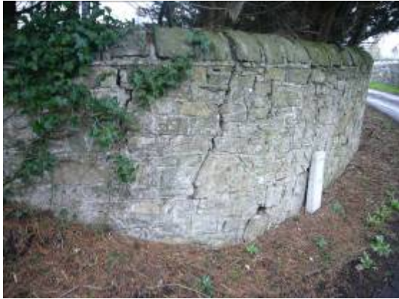
Stone boundary walls are a feature of the area. This wall appears stressed by the proximity of fast growing trees.
