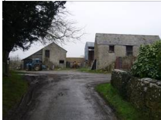
Llancadle Farm's outbuildings form a good collection of historic vernacular farm buildings. Some are in need of repair.
