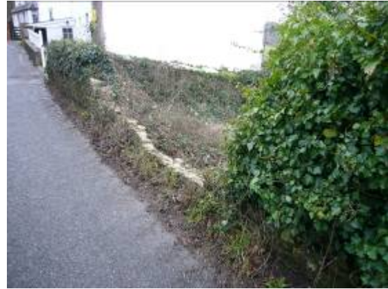
Part of the stone wall beside The Manse has collapsed and is in need of reconstruction. The adjoining field is in poor condition.
