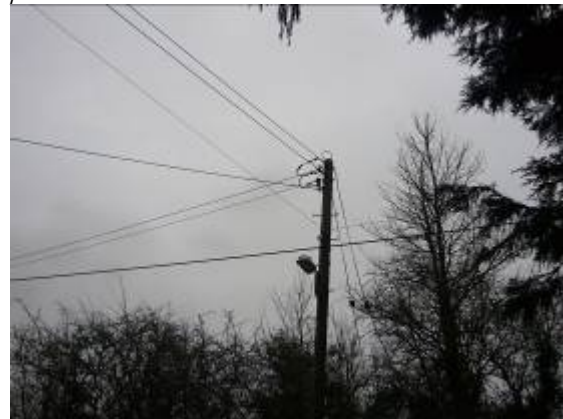
Wires and cables intrude upon the streetscene.
