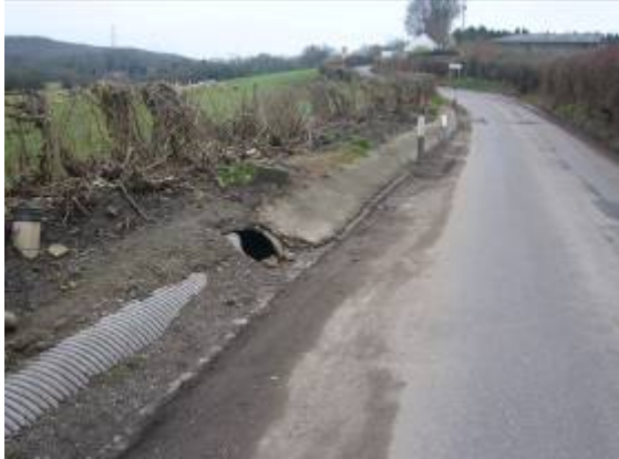
The culverted stream beside the approach from Greenway is in need of repair.
