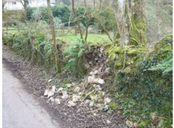
Stone walls have collapsed in places.
