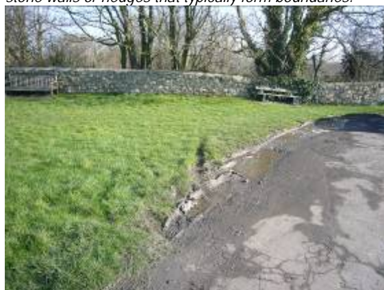
Car parking by the green is eroded the unkerbed grass verge.
