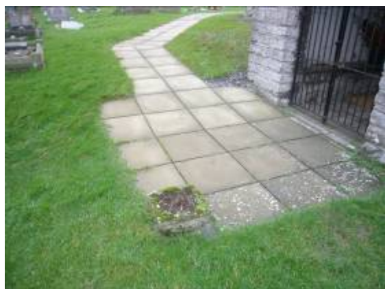
Concrete slabs are a poor quality surface for the approach to a medieval church.
