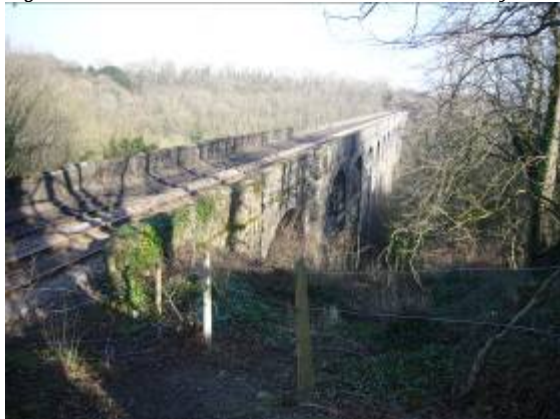
Porthkerry Viaduct, a grade II listed building outside the conservation area, is a local landmark.
