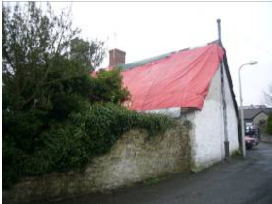
Lower Farm Cottage is in need of re-thatching.
