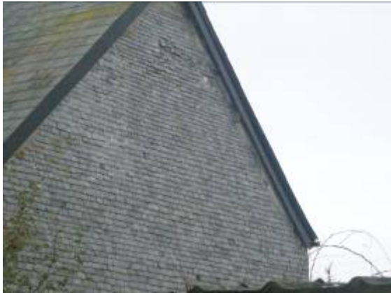
The exposed west gable of Lower House farm is given extra protection by slate hanging.
