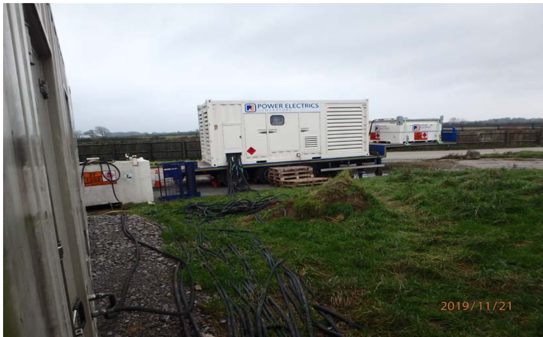
Photo 3. - temporary operational generator - located to south-west of Hangar A.
