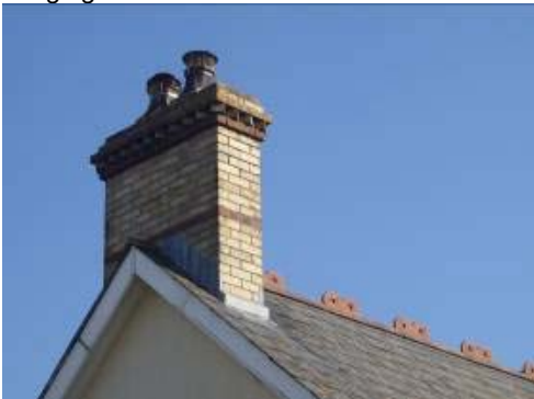
Chimney stack embellished by two tones of brick colour and ornamental courses.
