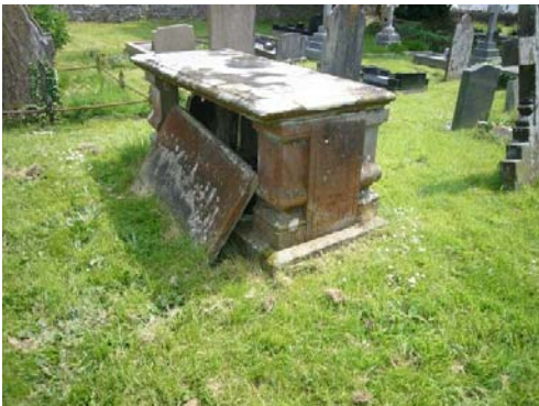
Tomb in need of repair.
