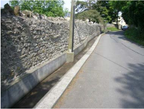
The concrete culvert of the stream by the church is stark and unsightly.
