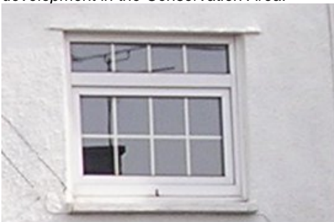
Some alterations, such as the insertion of plastic windows, dilute the character of the Conservation Area.
