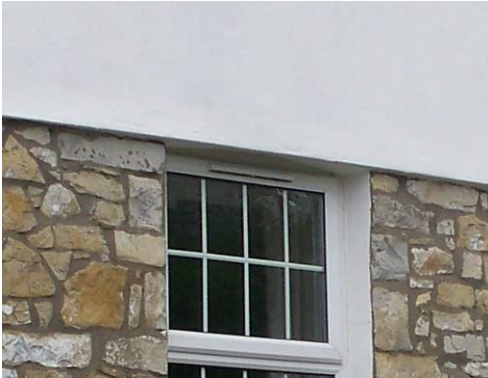
Here, inappropriate plastic windows and the stripping of render detract from the character of the area.
