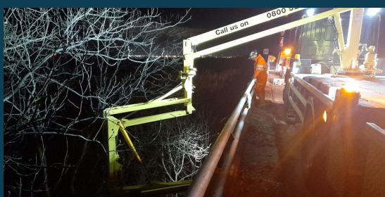
Serious access equipment required
