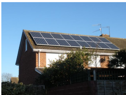
Example 1: Solar PV Panels
