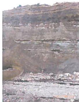
P2 - fallen blocks and debris
