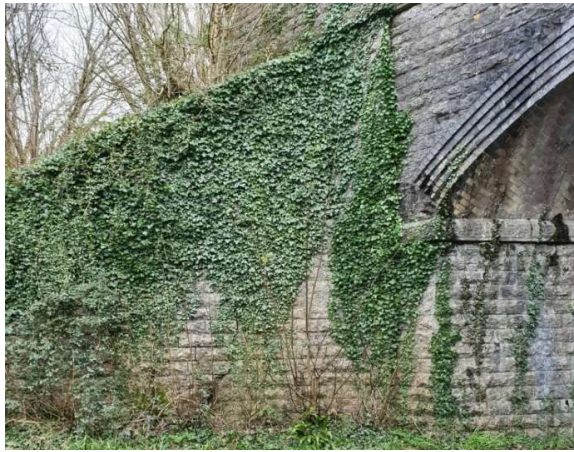
Figure 16 – Fort Road Wingwall – General Condition
