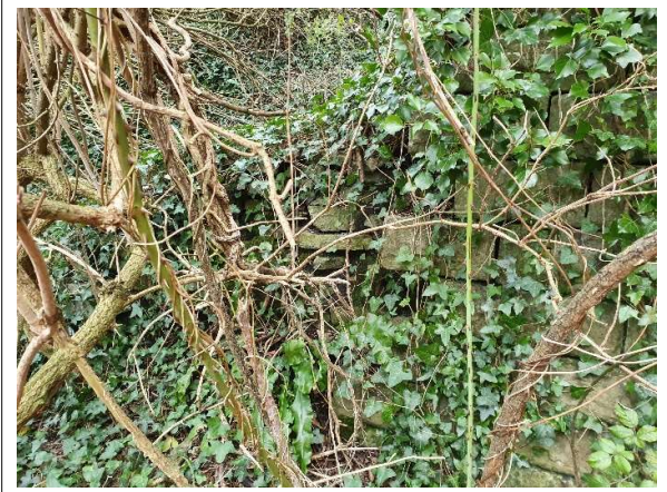
Figure 40 – Additional Structure 3 Missing Wingwall End
