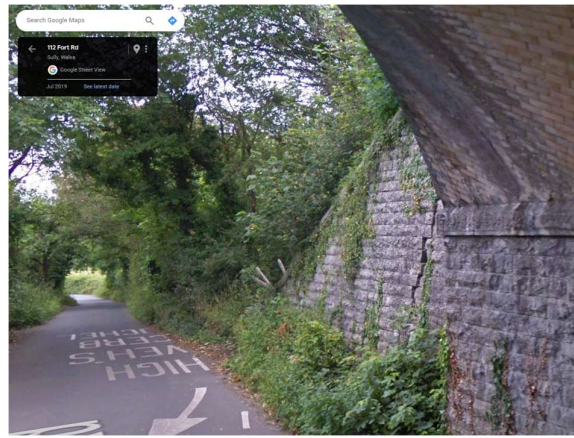
Figure 23 - Fort Road Wingwall Crack - Google Street View 2019
