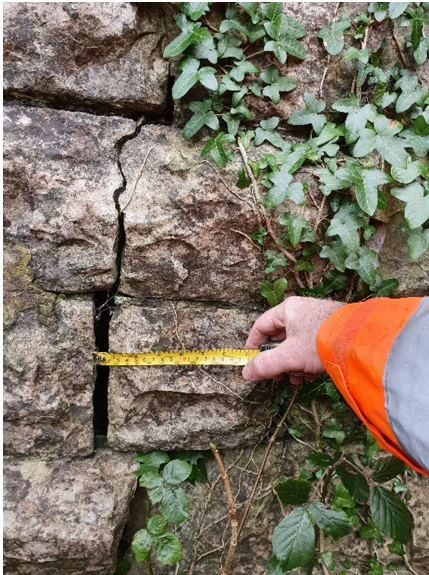
Figure 18 – Fort Road North Eastern Wingwall crack width (>20mm)
