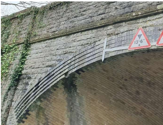
Figure 20 – Fort Road Evidence of Bridge Strike
