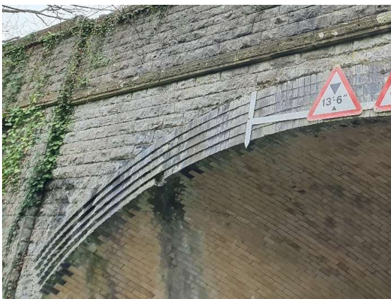
Figure 20 – Fort Road Evidence of Bridge Strike
